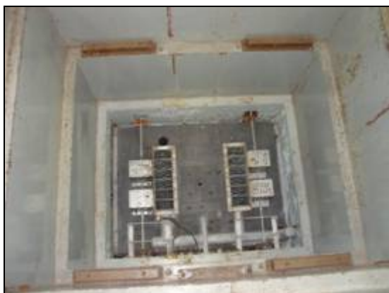
Core area showing fuel tanks, pipework, control absorbers and graphite (Oct 08)
