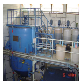
Chemical Precipitation System
