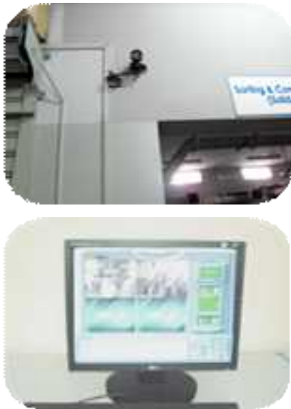
Figure 1: CCTV & Control Panel of Physical Security System at CWPSF
