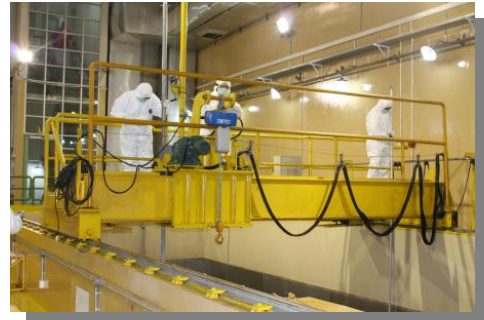
Fig1: Sliding Bridge of TC-ISFSF
