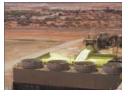
Copper Refinement Facility
