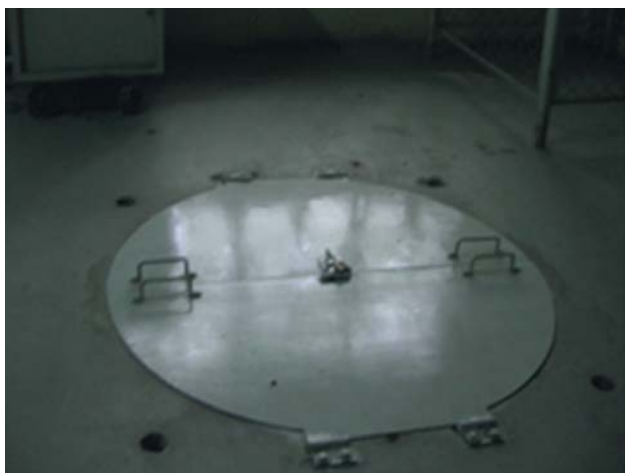
Access from the ground floor were sealed with steel plate and grills for security reasons
